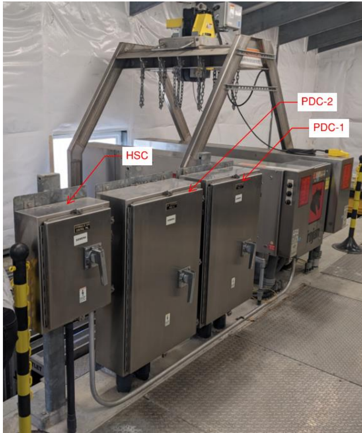
Figure 3-3 | Existing UV Panels
