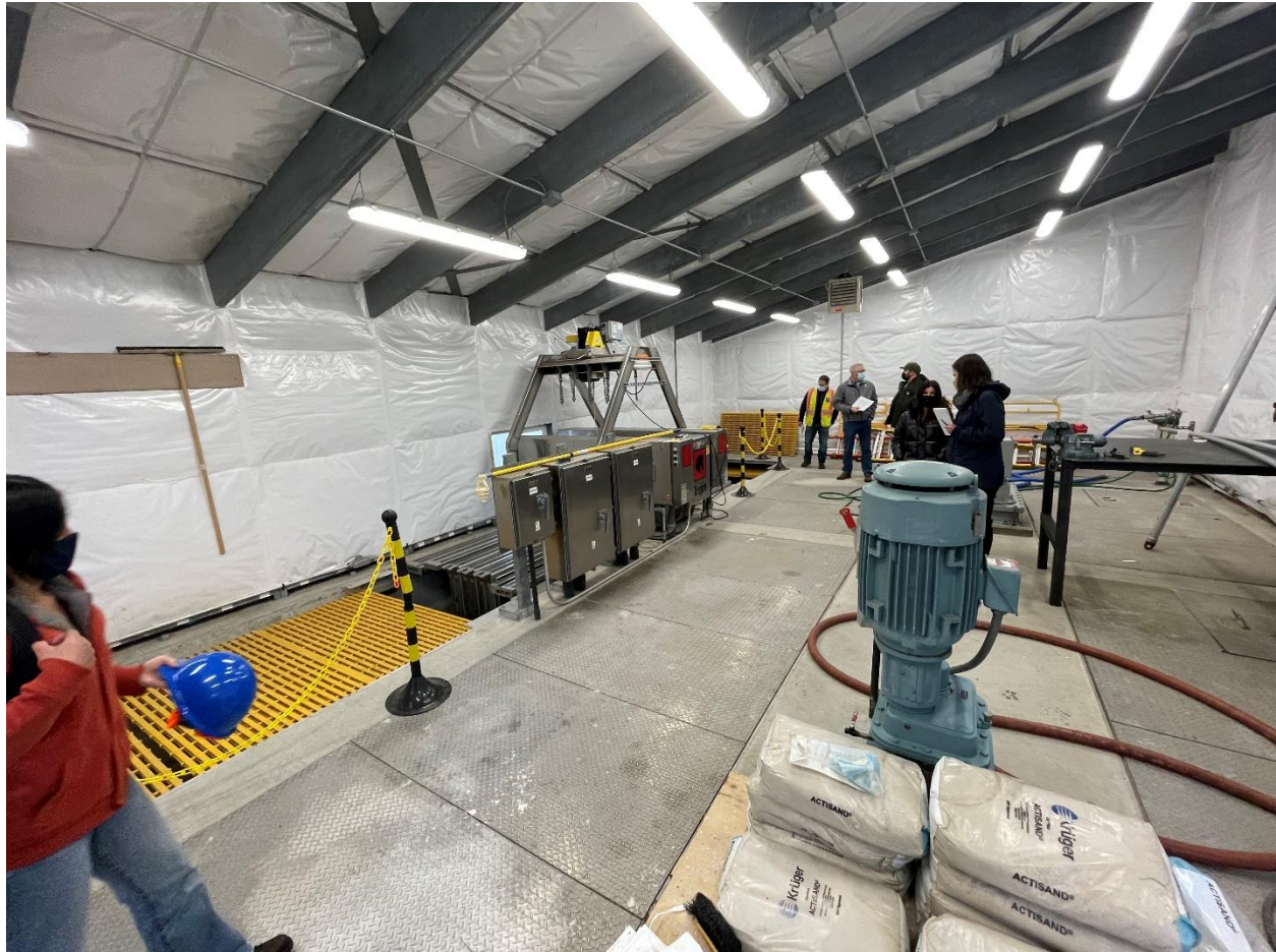
Figure 3-2 | Existing East Plant UV System
