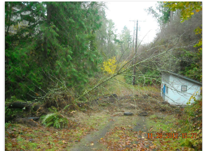
2012 landslide partially blocks access to existing pump station in Schley Canyon with mud and debris.
