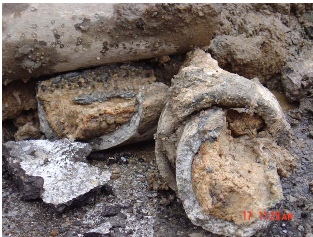
Grease buildup on interior of sewer line
